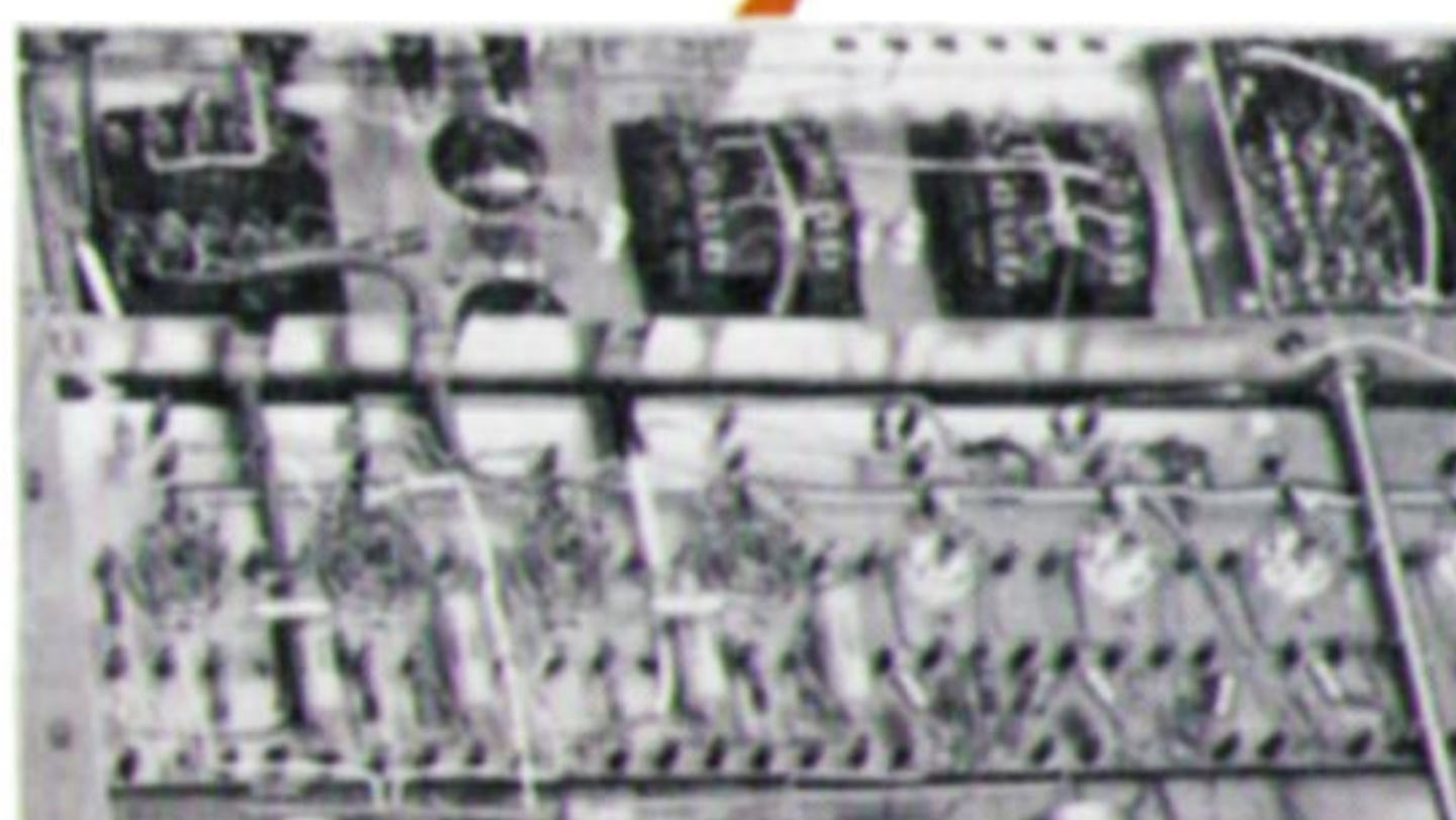
Immaculate wiring and high grade components ensure reliability and consistent performance.
